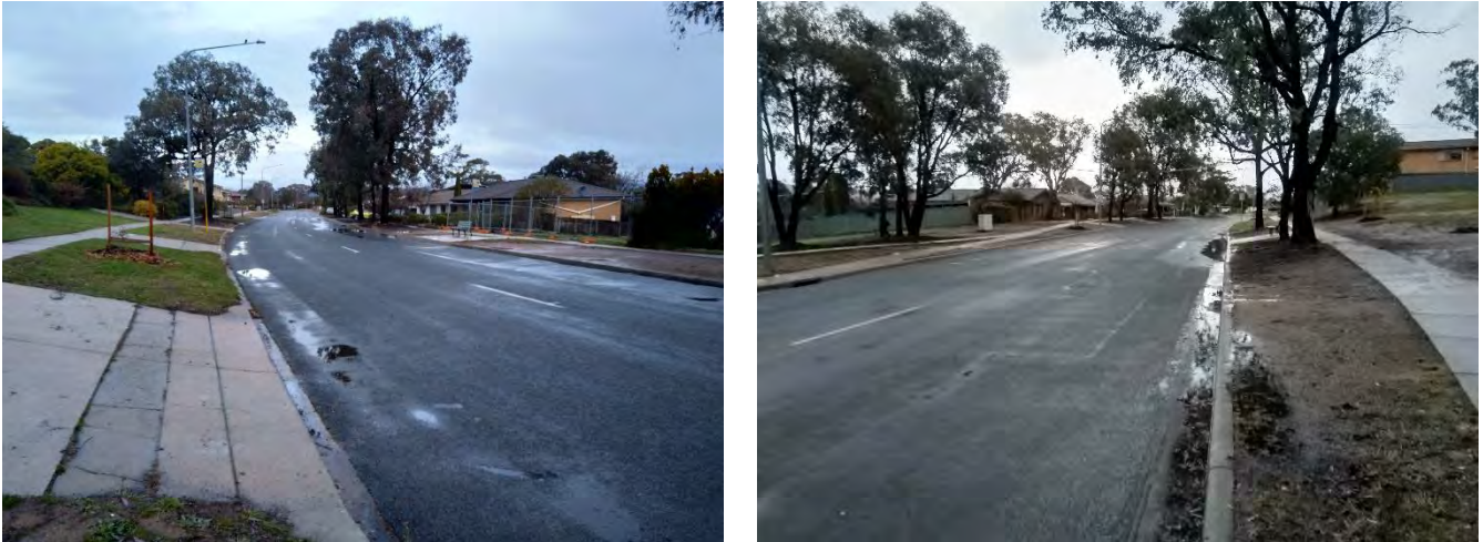
Figure 20 Water Ponding on Roadway
