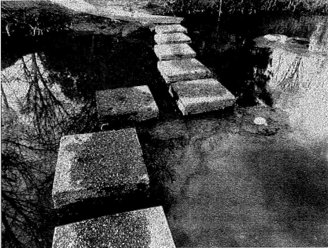
Figure 2-3 Photo 2: Gap between stones
