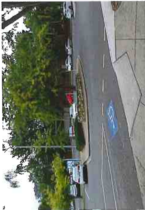
1 Disable carparks - non-compliant
