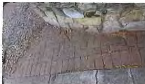
Cracked and tired pavements
