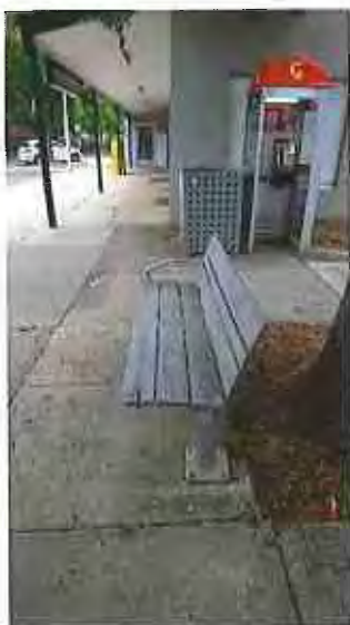
Eastern shops have greater than 1:40 cross fall and stepped entry
