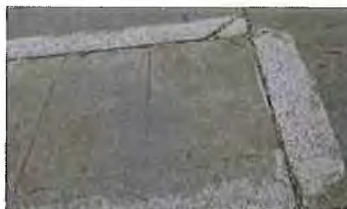
Cracked and uneven pavements
