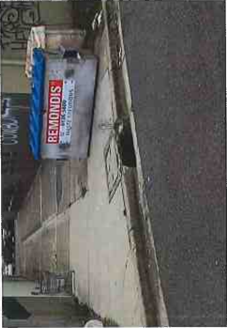
2 Damaged service lids
