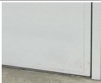
Metal faced and wrapped external doors – doors to be solid core with exterior waterproof plywood facing.
