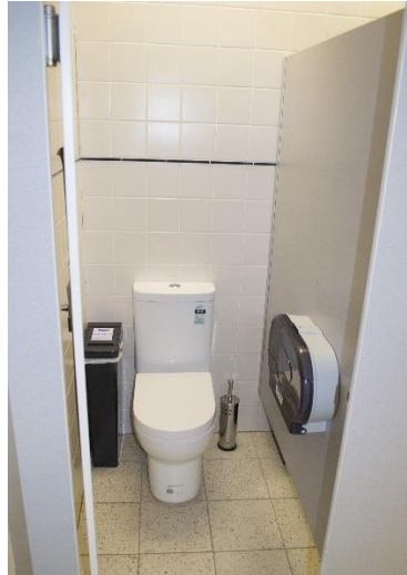
Non-stainless-steel fixtures and fittings – Not to be Used.
