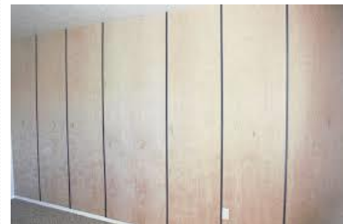
Unfinished walls – Not to be Used.
