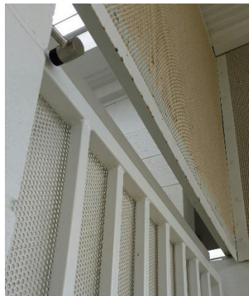
External mesh screens that are out of alignment – that have gaps that allow birds and vermin access – Not to be Used.
