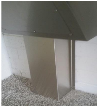
Stainless steel enclosure to all exposed services.
