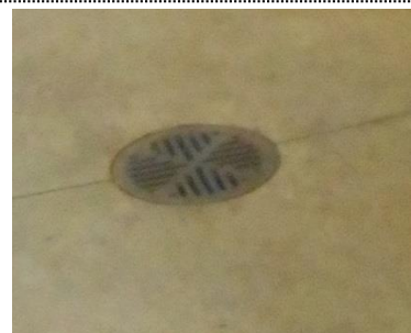
Floor wastes to be large bucket trap type with open grate for ease of clean-out.
