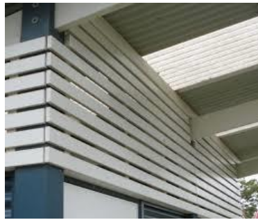
Battens over door head for natural light and ventilation into internal areas.
