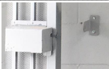
Metal gate with slide bolt / pad bolt and padlock in security shroud. Gates to be held open with wall mounted bar.
