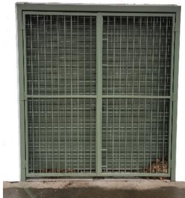
Roller shutter, with security gates pad bolts and padlocks.
