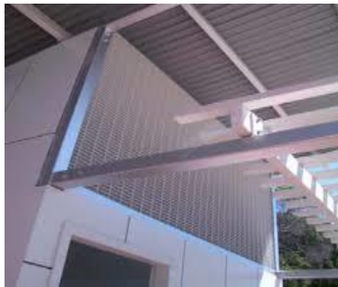
Perforated metal grilles over door head for natural light and ventilation into internal areas.
