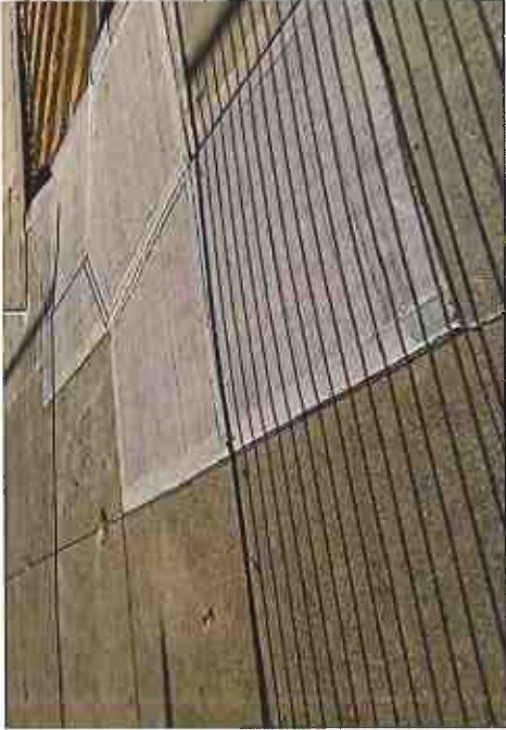
2 Old concrete paving
