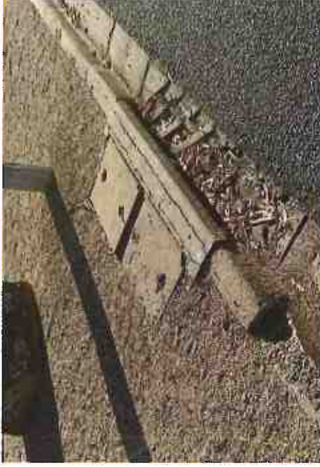
2 Damaged service lids
