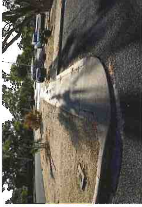
Non-compliant kerb ramps
