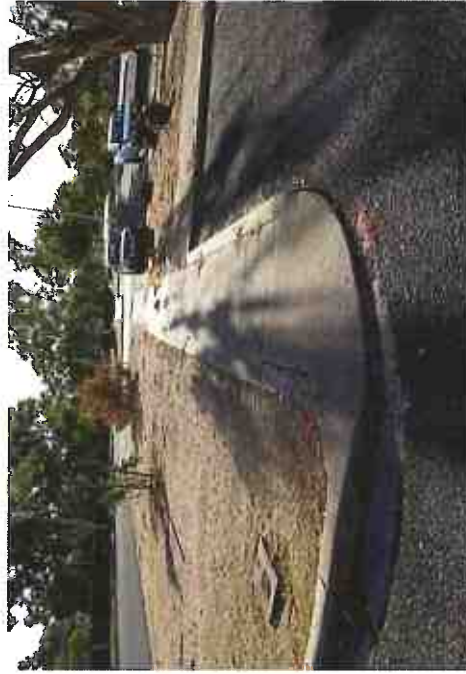
4 Kerb ramps require upgrading
