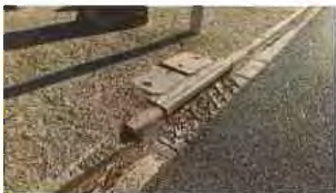
Damaged service lids and kerbs
