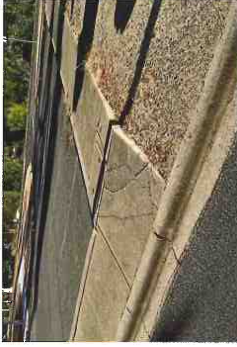
3 Badly damaged paving
