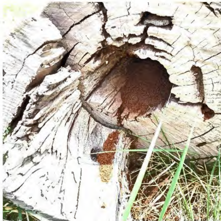
Image two: evidence of termite activity
