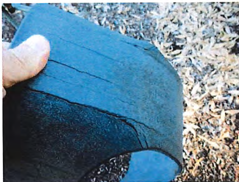
Photo taken: 25/05/2017 Toddler seat cracking. Monitor.
