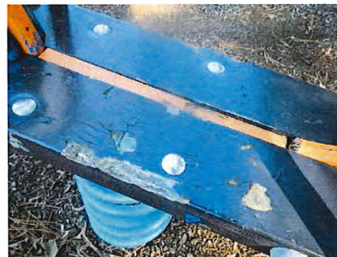
Photo taken: 23/05/2016 Peeling coating, monitor.
