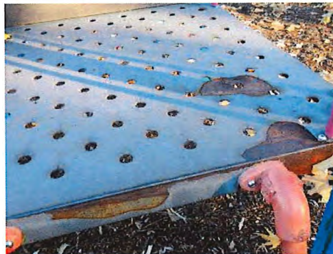
Photo taken: 25/05/2017 Deck coat peeling. Monitor.
