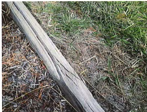
Photo taken: 03/05/2011 Some sections of timber edging exhibit splitting. Monitor.
