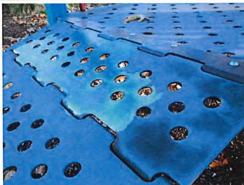
Photo taken: 25/05/2017 Clatter bridge coating peeling, monitor.
