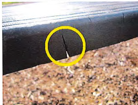
Photo taken: 01/05/2012 Small split in edge of flat seat. Monitor.
