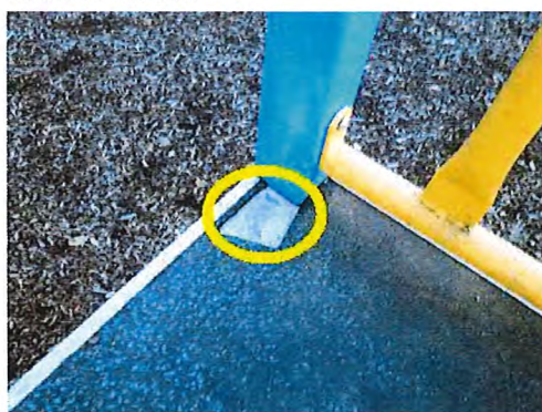
Photo taken: 13/05/2010 Coating cut off deck. Monitor.
