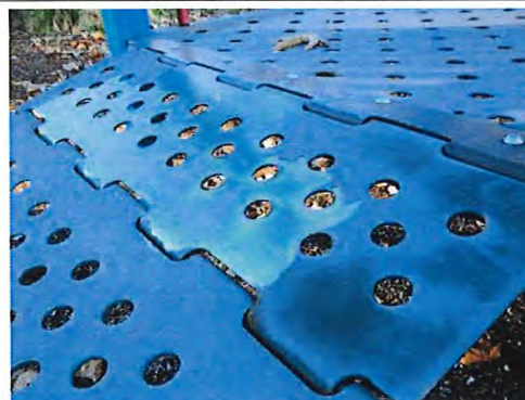
Photo taken: 25/05/2017 Clatter bridge coating peeling, monitor.
