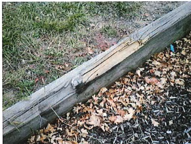
Photo taken: 03/05/2011 Some sections of timber edging are splitting. Monitor.
