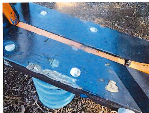
Photo taken: 23/05/2016 Peeling coating, monitor.
