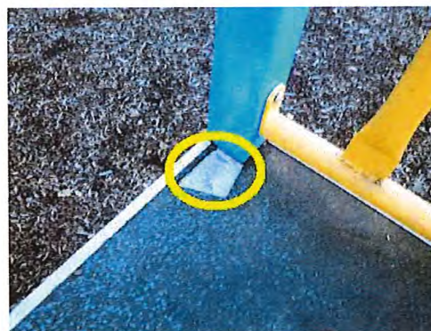
Photo taken: 13/05/2010 Coating cut off deck. Monitor.
