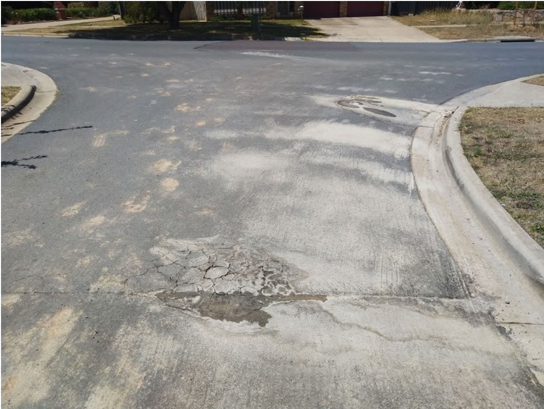
Plate 1: Crocodile Cracking and seepage from pavement.
