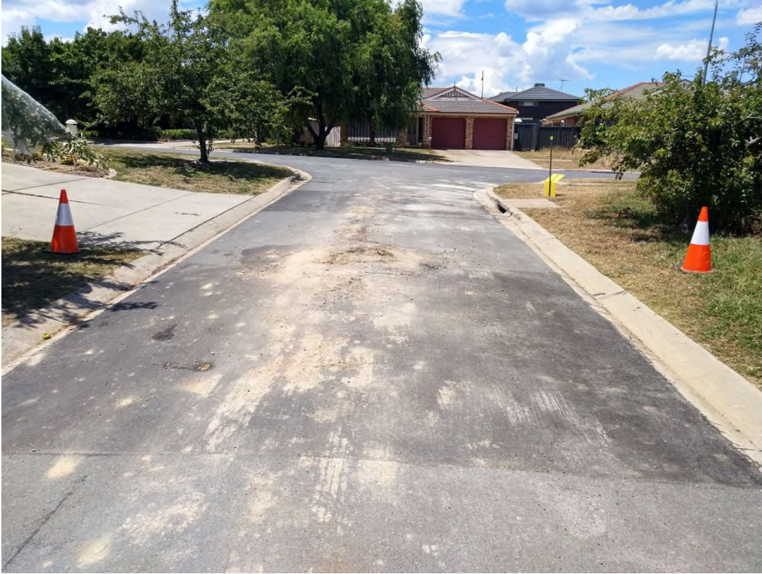
Plate 2: Major pavement failure.
