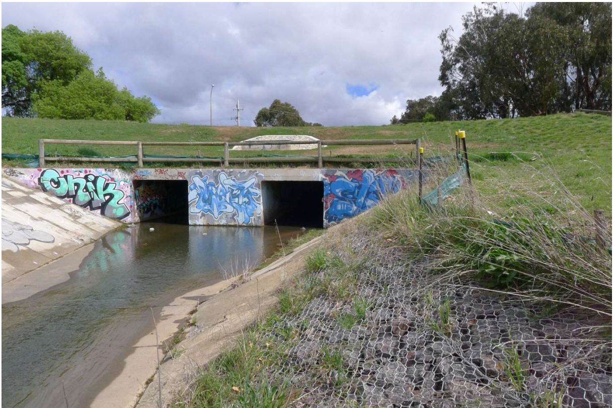
Figure 2-2 Southwell Park low level outlet culverts (looking downstream from the gauging pond)
