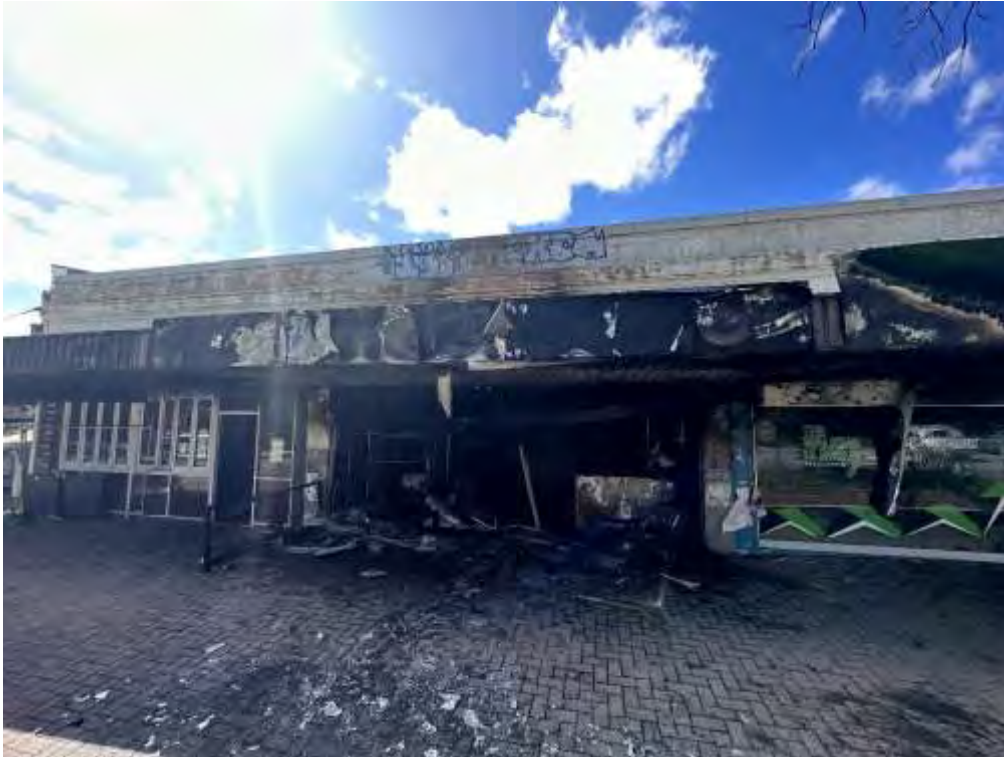
Image 3. View of the shop fronts of the fire damaged property
