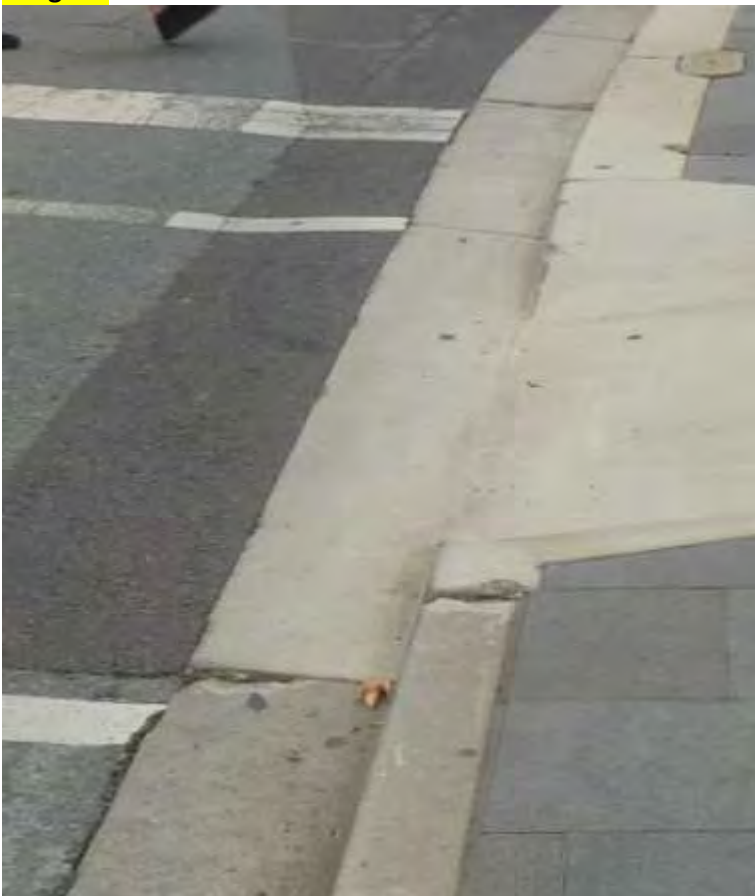
A typical transition done at crossing point or driveway between the 150mm and 300mm wide top kerbs. Image-5.
