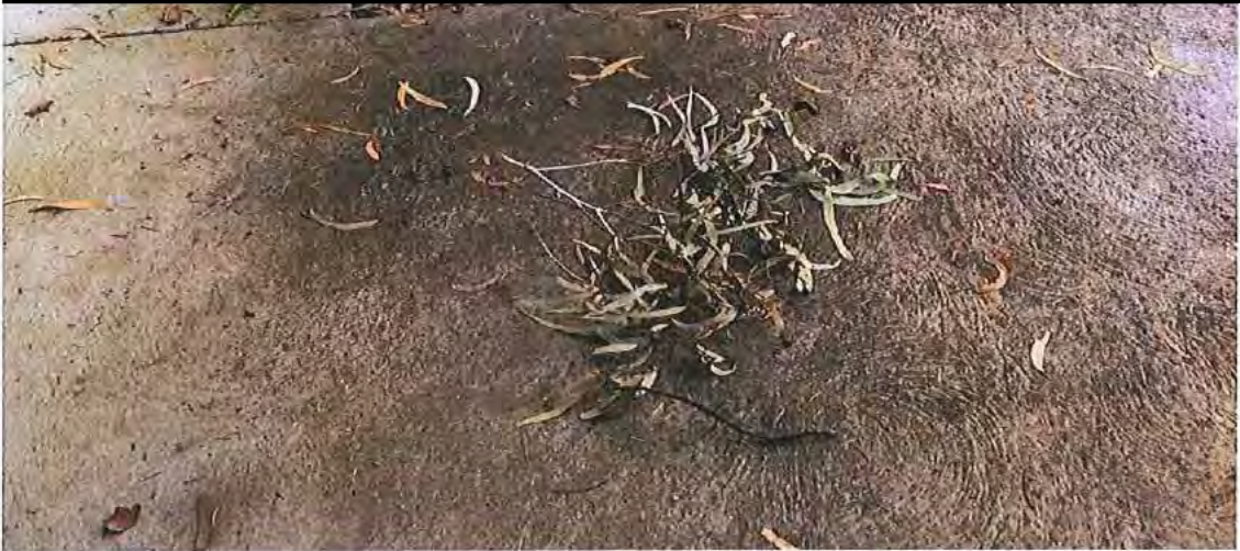
Figure 14: Stained Concrete from Tree Litter (31 Jan 22)
