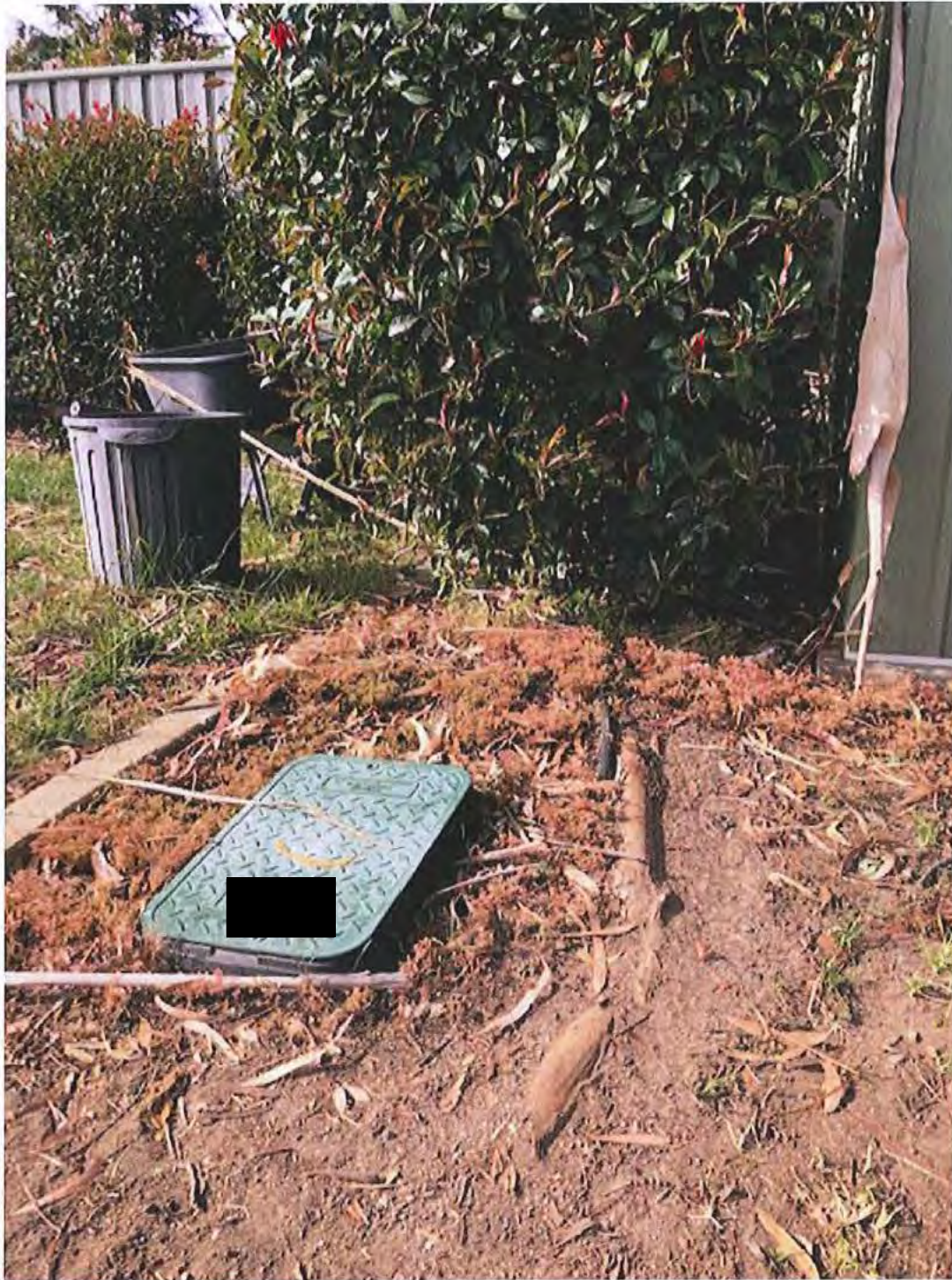
Figure 20: Encroaching Roots Near Infrastructure (6 Feb 22)
