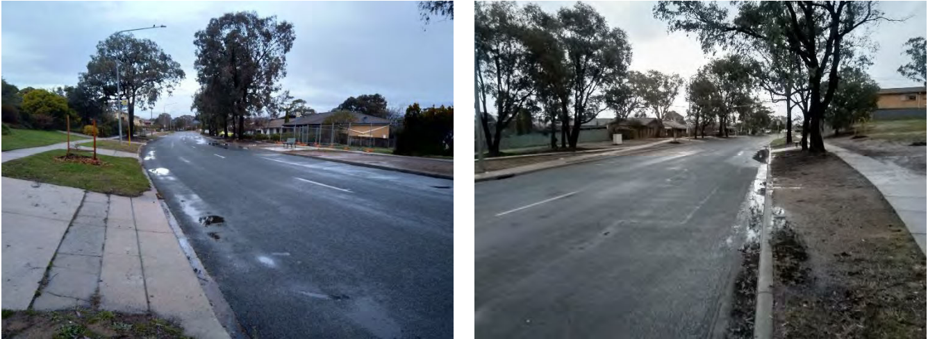
Figure 20 Water Ponding on Roadway
