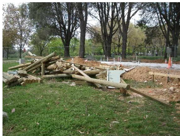
Figure: Demolished site of toilet block October 2010 (Source: SMM)
