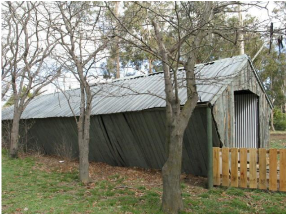
Figure: External eastern side of tunnel. Damage visible.
