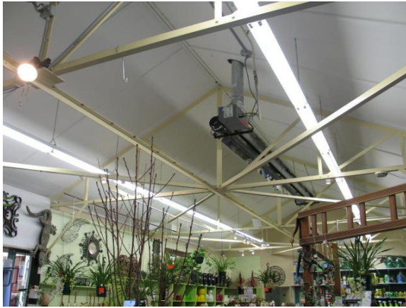
Figure: Internal view of older western structure, showing steel construction and clad roof.
