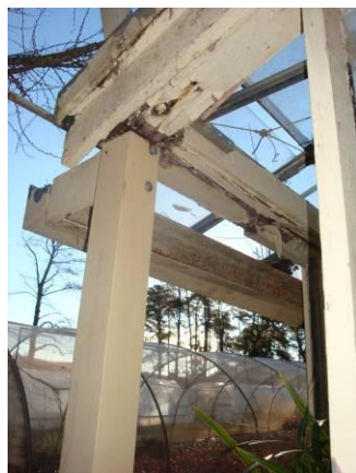
Figure: External guttering attached to timber frame. Poor condition visible.
