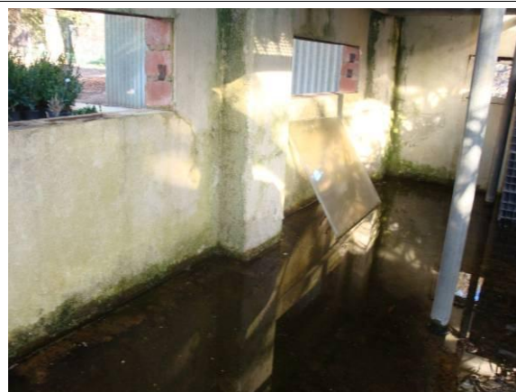
Figure: Water collecting at southern end of glasshouse no. 34. Ventilation holes visible.
