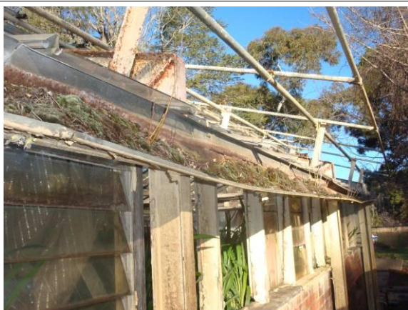
Figure: Gutter damage on western wall of glasshouse no. 34.
