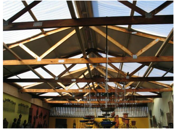
Figure: Internal view of middle structure showing timber construction and Perspex clad roof.
