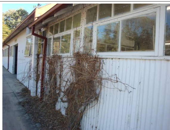
Figure: View of vines causing damage to external walls.
