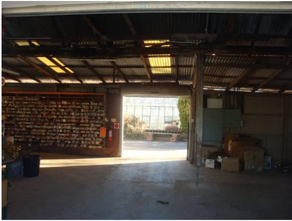
Figure: Interior of Dispatch Preparation looking west. Steel base visible on structural column.
