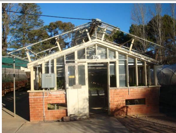
Figure: Glasshouse no. 34 showing steel frame construction over the top of timber roof.
