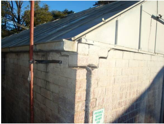
Figure: Wall damage visible on glasshouse no. 24.
