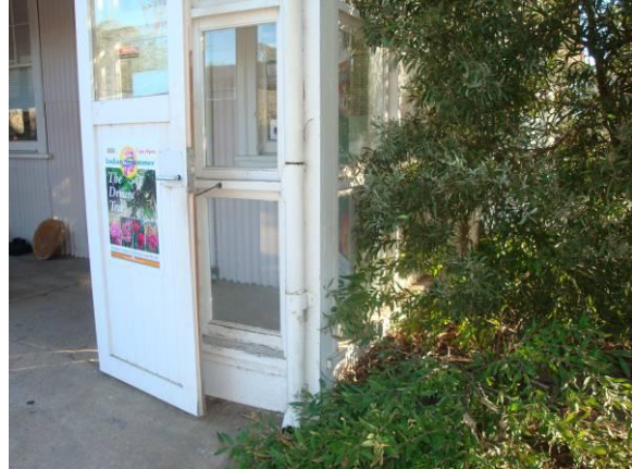
Figure: Front entry door, with vegetation build up against north wall.
