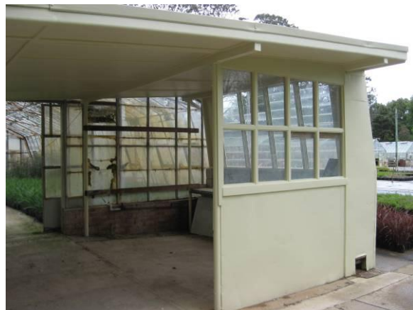
Figure: Newly restored workshop end of building. Access to glasshouse no. 6 at rear.
