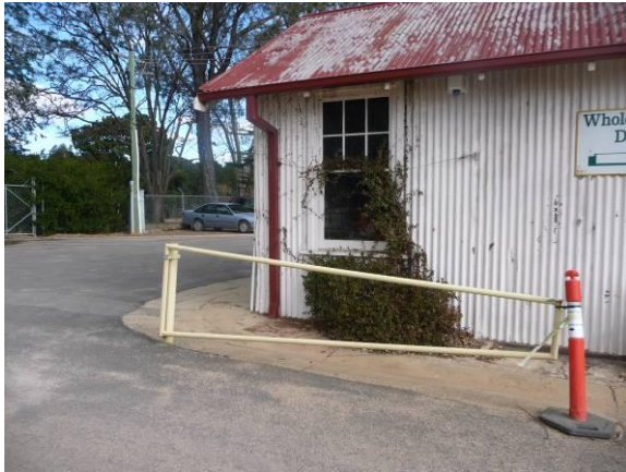
Figure: Southeastern corner of Dispatch Preparation building, showing vegetation damaging window.
