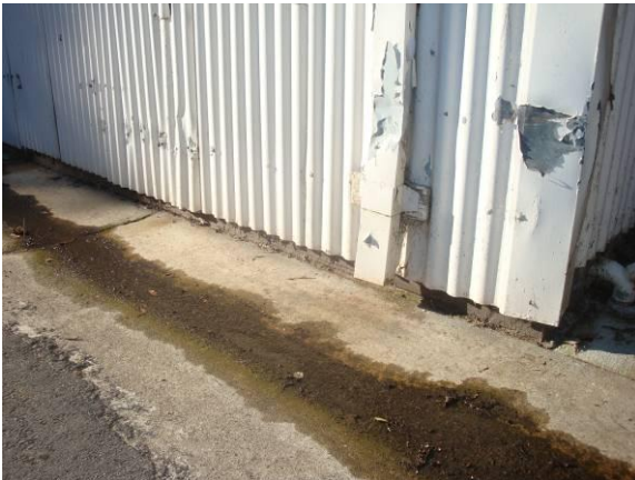
Figure: Damage to lower walls visible, drainage issues.
