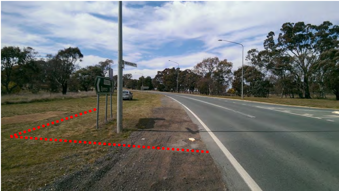
Photo 4.1: Kuringa Drive at the T-intersection with Owen Dixon Drive, looking East. Ruts, pot holes and wheel tracks can be seen on the left hand shoulder where cars have been travelling to overtake vehicles turning right into Owen Dixon Drive.
