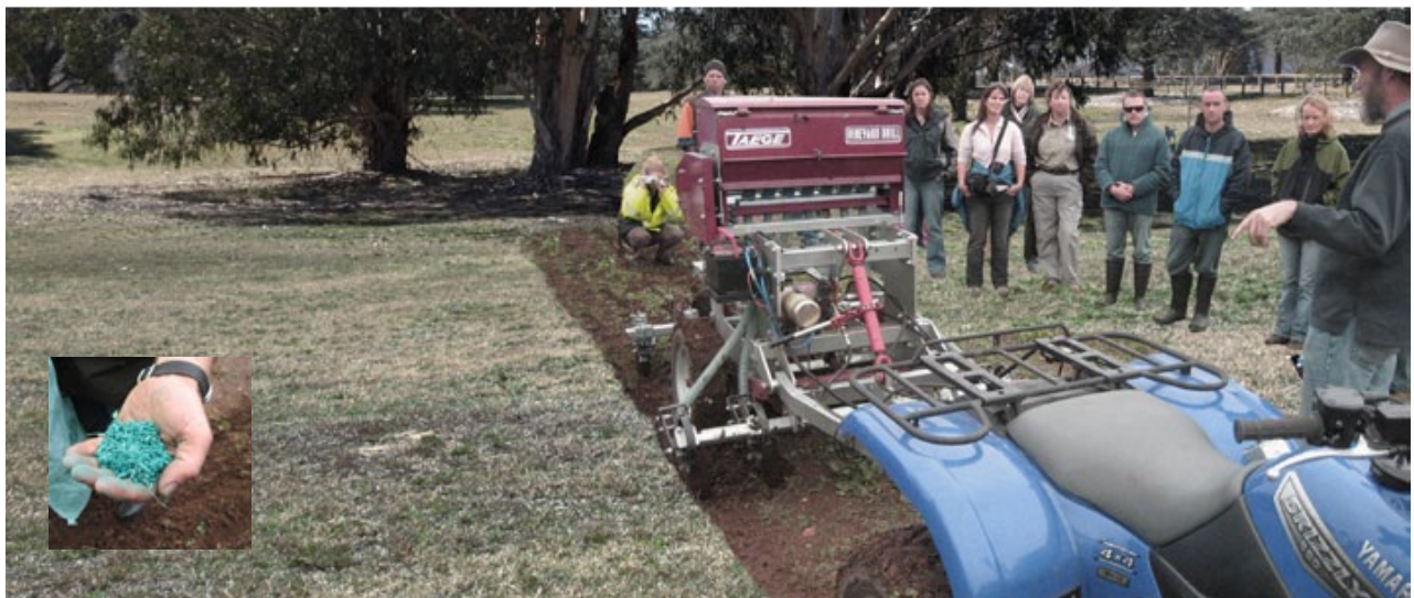
Dryland grass areas in the northern and eastern parts of Weston Park are rehabilitated as native dryland grass meadows suitable for recreation. Direct seeding techniques will be tested and may have broader application to other similar areas within the Canberra Open Space System. Images Oxygen
